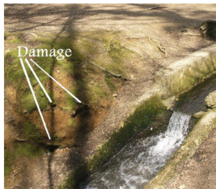
Damage to Dam and Spillway at Waggoners Wells
